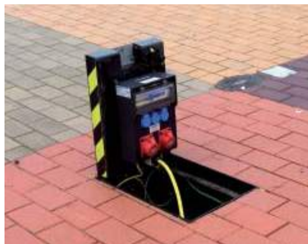
Additional in ground power supply as needed
