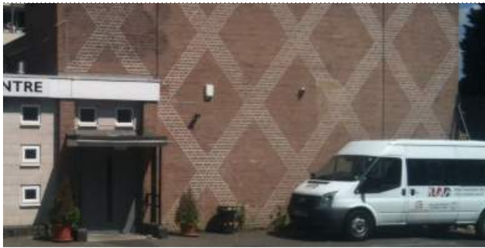
Example of a graphic applied on a brick wall using pointing colour
